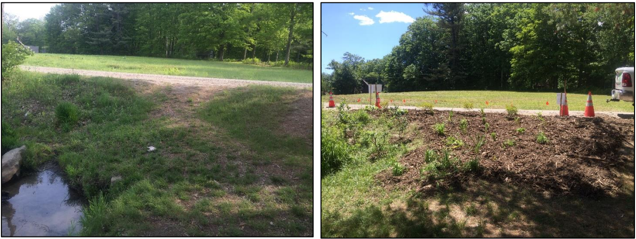
Before (left) and after (right) condition of vegetated buffer along Pine Cliff Road.
